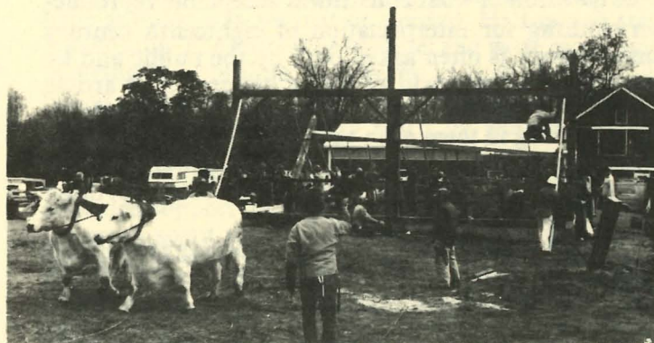
Oxen and Human Power Raise the Second Bent of the Saunders Barn
