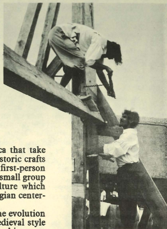
Isaac Allerton House, Plimoth Plantation August 1973. Dr. Henry Glassie, folklorist, instructs his volunteer helper, Joseph Saviola, how to drill a 1627 hole with a circa 1875 twist bit auger. The house plan is based on Henry Glassie's field work in the British Isles.
