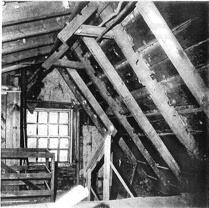
East gable of house, original Stage I pit-sawn rafters. Stage II rafter boarding and Stage III window and infill. Intermediate rafters added in Stage IV
