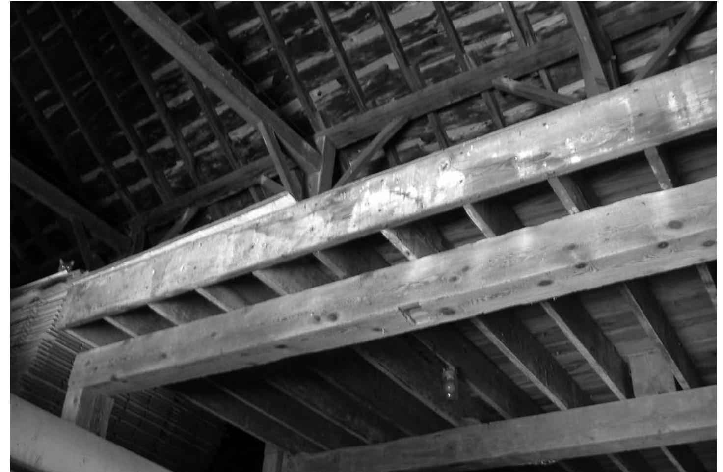
Top of H-frame post appears with upper tie beam and tie brace. At top of post are purlin plate and its braces. Above purlin are rafters.
