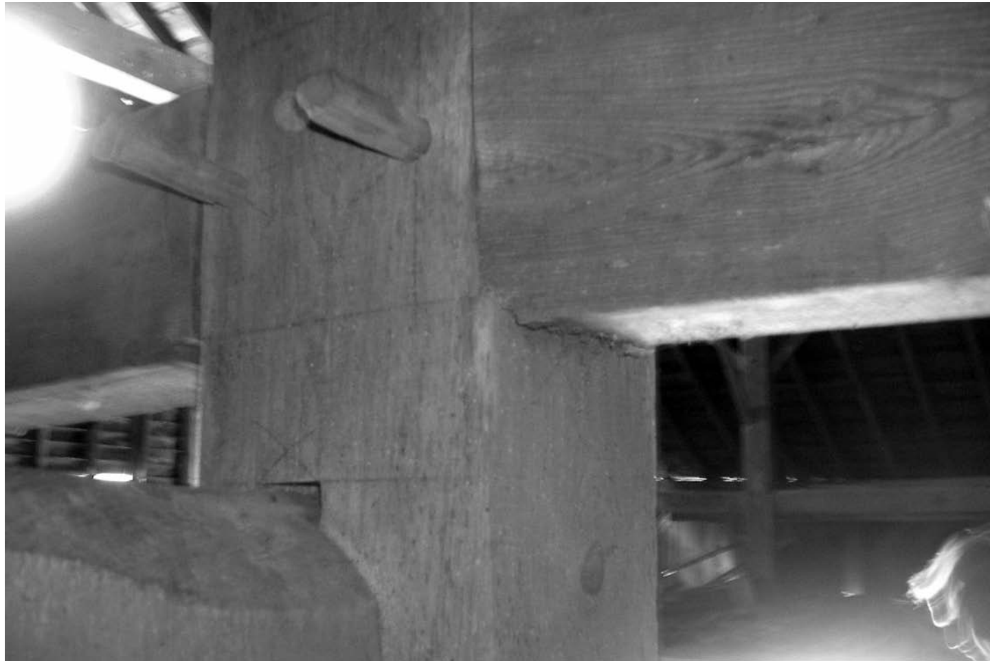
Two beams seen at bottom half of photo are likely the recycled anchor-beams.
