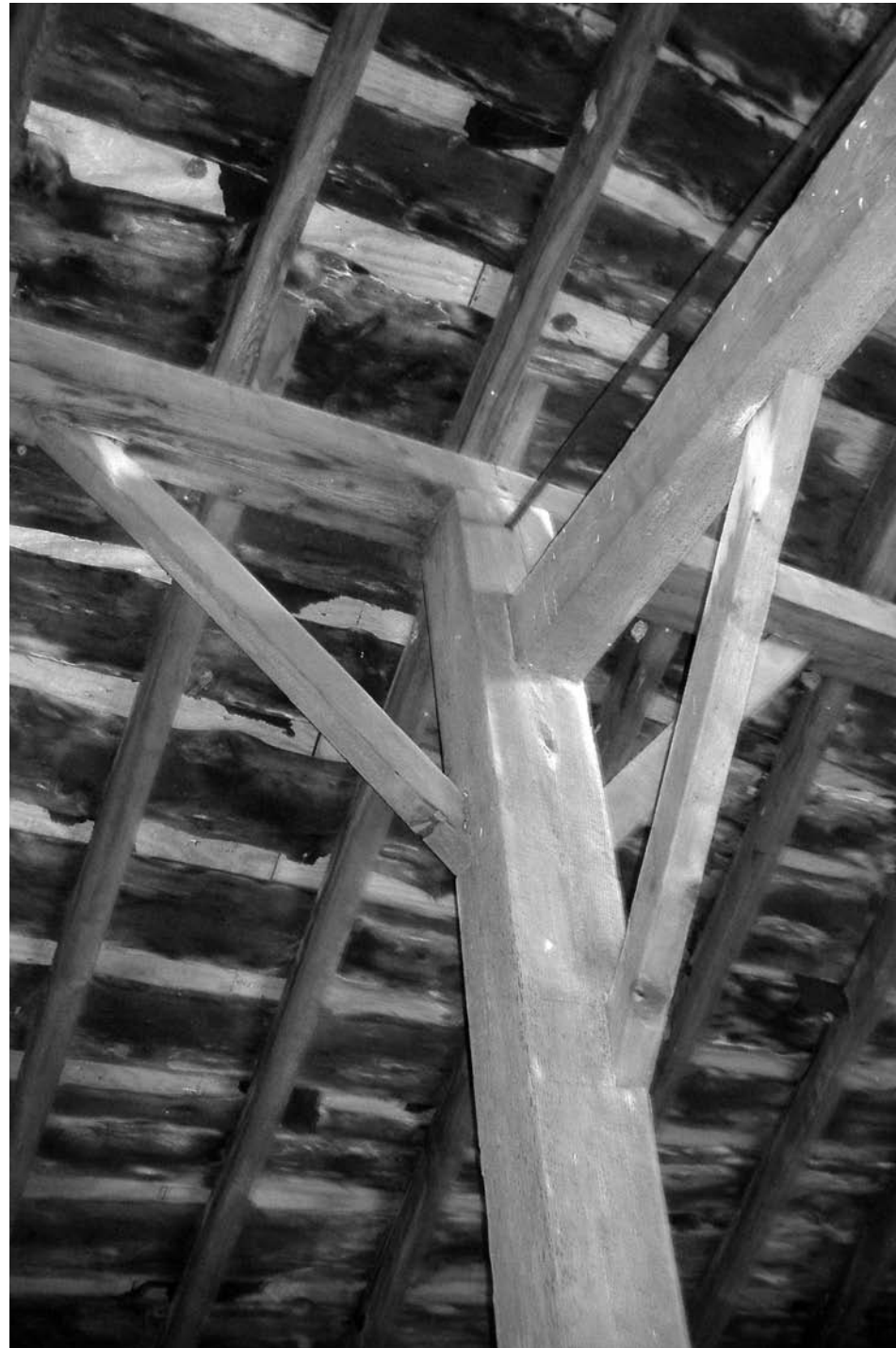
H-frame post is joined to high longitudinal ties. At lower left is a high side aisle tie. Pencil marks to denote placements of mortises are easily seen.
