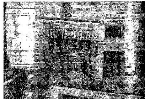
You can see all the work that is being done. Peter and I did not go into the house due to all the construction.
