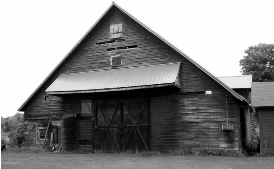
View of front gable wall of pre-Revolutionary War era five-bay Bruyn-Mahoney barn, with classic roof proportions (on Rt. 209 near Wawarsing, in Ulster County). The barn has new metal roof and sill system. Cladding is not original. Exterior dimensions are 50' at each gable wall and 60' at each side wall.
