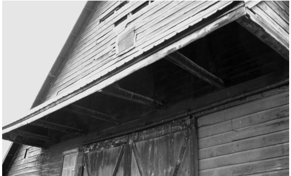
Close-up view of original pentice at front gable wall of the five-bay Bruyn-Mahoney barn in Ulster County. Note seven original hewn pentice arms that extend beyond wall by just over 5'. Pentice arms originate from first interior anchorbeam and stretch over the gable wall anchorbeam to the exterior.
