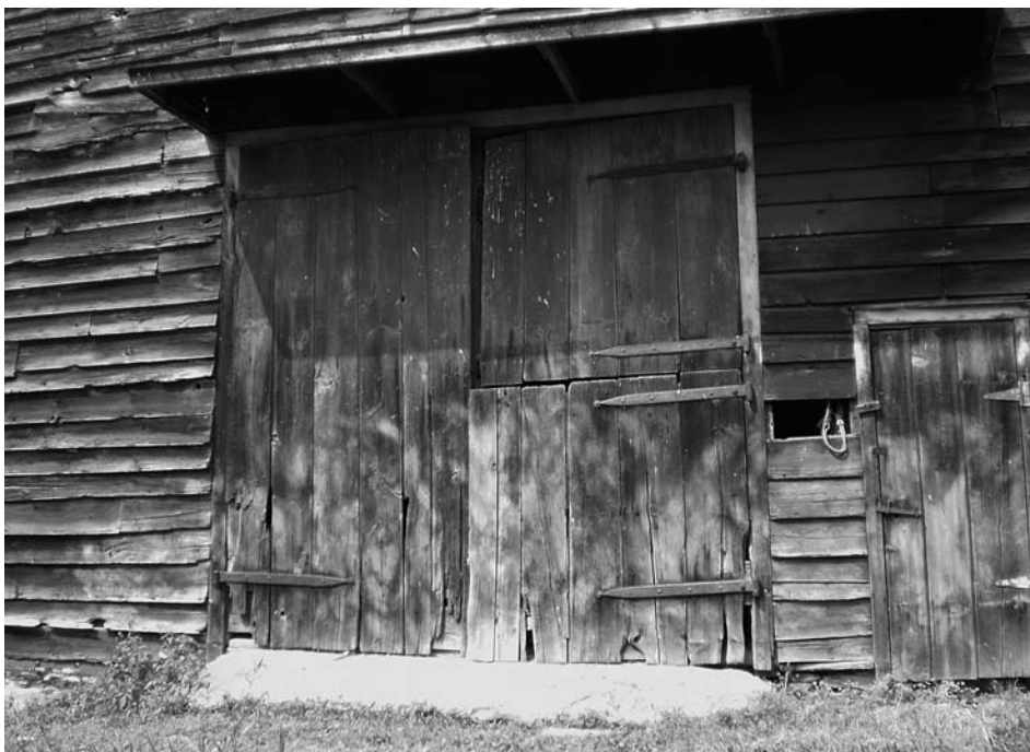
Colluci side wall entry English barn near Gardiner in southern Ulster County with three section nearly original wagon doors. Full height door appears at the left and two half door sections are seen at the right. Pentice is seen over the wagon doors.
