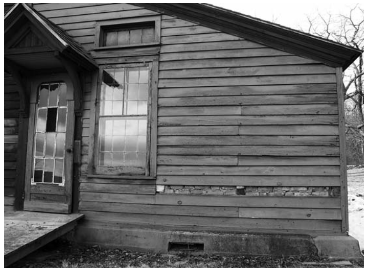
The lean-to additions on either side of the Brandow house appear to be built soon after the main section as evidenced by the exposed brick noggin seen here in the north addition.
