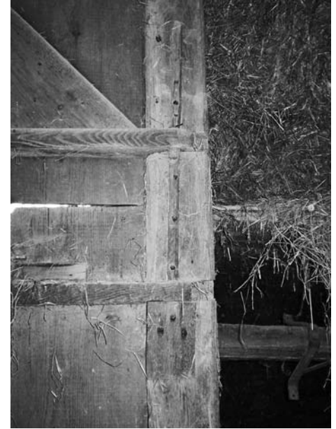
Interior of John Snyder barn and view of very long single piece wood pintle at right side of door opening that secures one wooden hinge of each of two half door sections.
