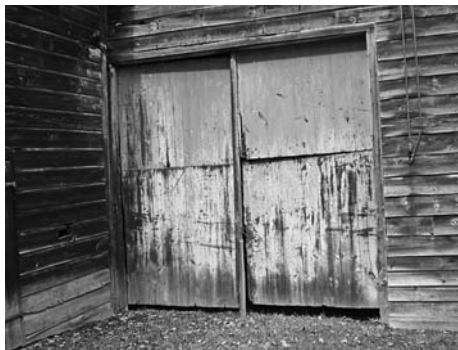
Replacement wagon doors at the Oliver 3-aisle barn in Marletown in Ulster County on south side of Route 209. Wagon doors are in four parts – two sections at left and two sections at right side. Doors swing inwardly that is likely not common for replacement doors in barns.
