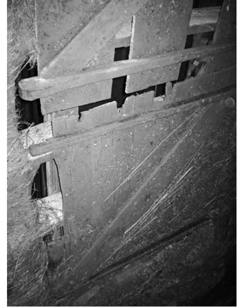
Two end wall wagon door sections seen on loft of dated 1766 Nieuwkirk barn on Hurley Mountain Road west of Kingston in Ulster County. Note original wooden door hinges.
