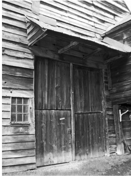
Original end wall wagon doors at the circa 1790 Bogart three-aisle four-bay barn in Marbletown, Ulster County, New York. Doors are in four half sections – two at one side and two at other side. Note mittelmanse at outside of doors. Above doors is partially original pentice.
