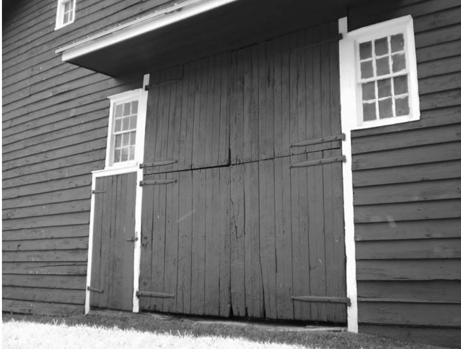
View of original end wall upper wagon door section at north side of door opening at the dated 1851 Elmendorph variant U-barn on route 213 near High Falls in Ulster County. Wagon door has two upper and two lower door sections and doors swing outwardly.
