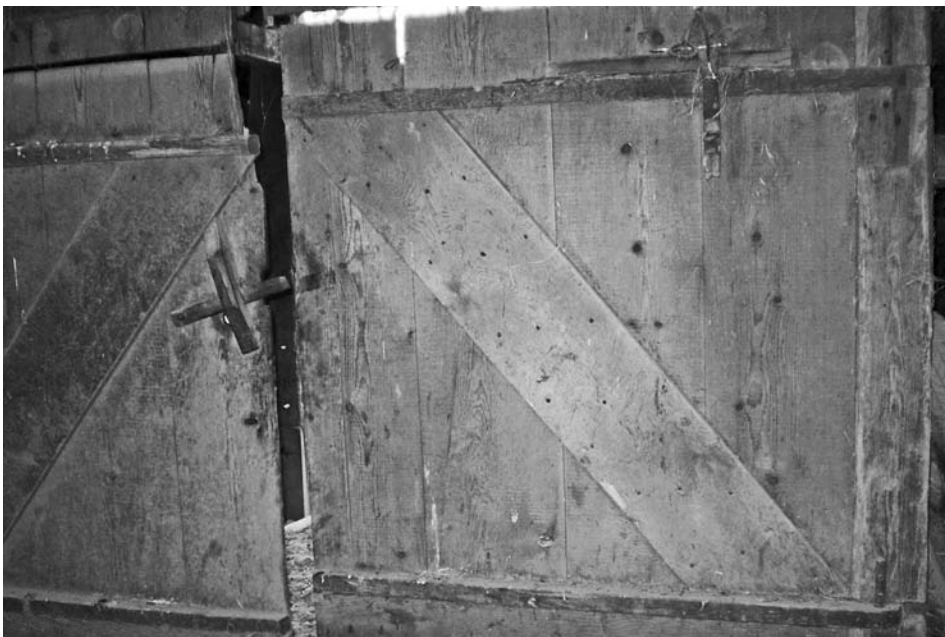
Interior of John Snyder circa 1820 side entrance Dutch-Anglo barn on Route 212 west of Saugerties in Ulster County. View is shown of two lower half door sections with wooden hinges. On left door is two-piece door latch.
