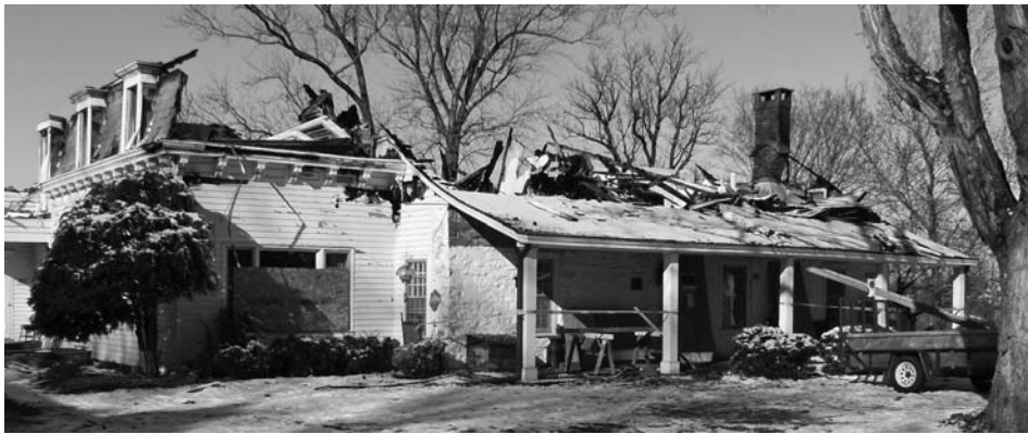
The Benjamin [a.k.a. Cornelius] Hasbrouck house after the devastating fire that occurred on Dec. 29th, 2009. Courtesy of the Historical Society of Shawangunk & Gardiner.
