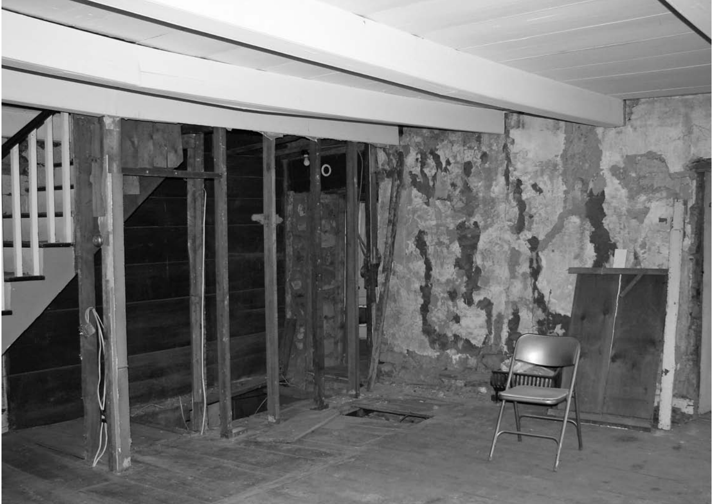
Fig. 2 – View from NE corner of north room during dismantling. Photo by Ken Krabbenhoft.
