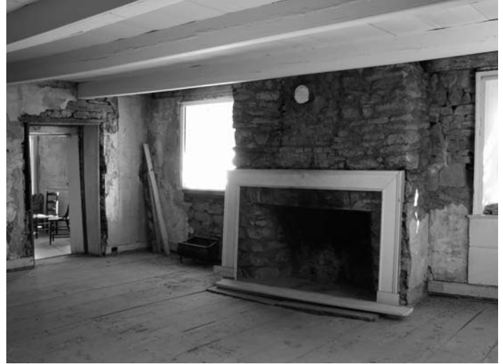
Fig. 8 – View of fireplace on north wall during dismantling. Photo by Ken Krabbenhoft.
