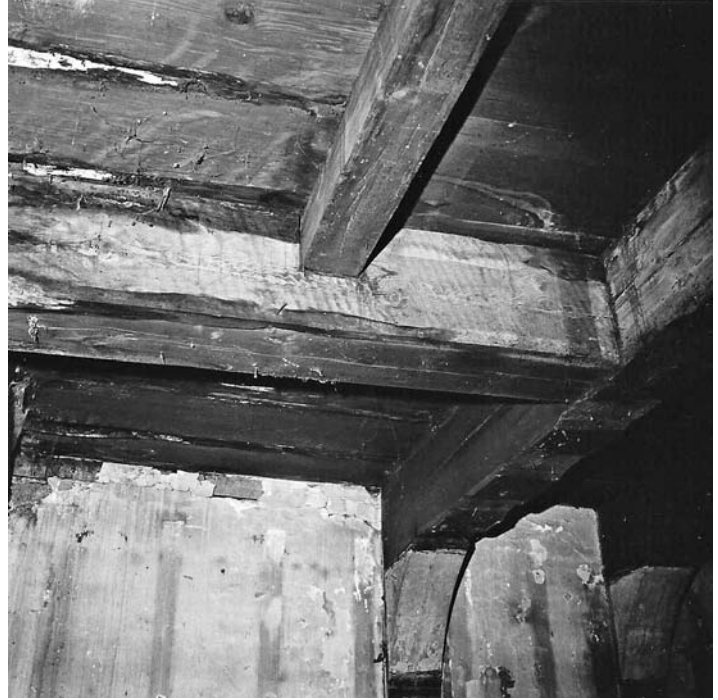
Fig. 11 – Inside (north side) of the south trimmer of the first floor fireplace at the east end of the North House. Note the kerf marks of a water-powered saw on the timber, and near its west end, the ghost of a wooden hanger that had carried the drop hood. October 1969.
