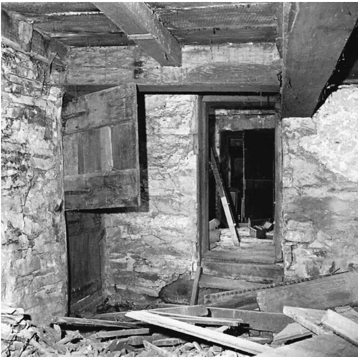
Fig. 6 – Basement of the North House, looking towards its south-east corner. Note the stain on the north face of the hearth trimmer from the iron hanger for the lintel of a basement fireplace. Note also the indication of the curvature of the trimmer arch that had supported the hearth of the first floor fireplace. The doorway at the right leads into the 'hyphen' and beyond there is a doorway into the basement kitchen of the Coeymans mansion. Both of these doorways are part of the late 18th century reconstruction of Coeymans. October 1969.
