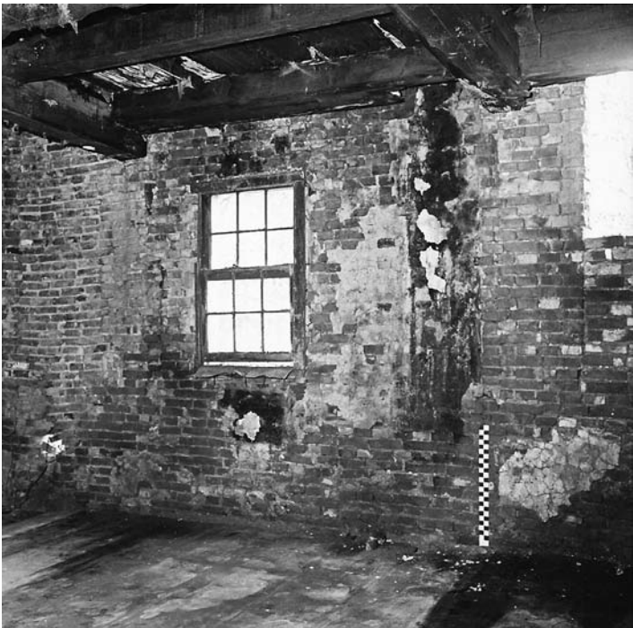
Fig. 10 – Interior of east wall of the North House, first floor, showing the central part of the wall. Note the sooty area that had been whitewashed over when the basement and first floor fireplaces were removed some time in the 18th century. There was clear indication of where the drop hood side members were housed in the brick. October 1969.
