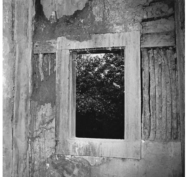
Fig. 3 – Interior of east wall of the 'connector' showing a window frame. Note infill with vertical sticks. September 1969.
