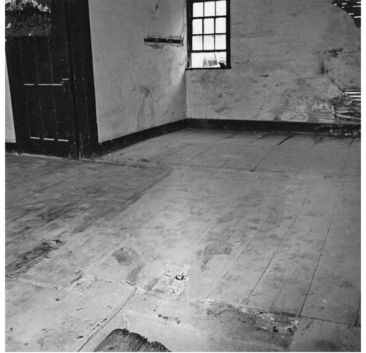
Fig. 7 – Interior of the first floor of the North House looking towards its south-west corner. Original flooring is shown. The closet door and lath-and-plaster walls are work done in 1878. October 1969.
