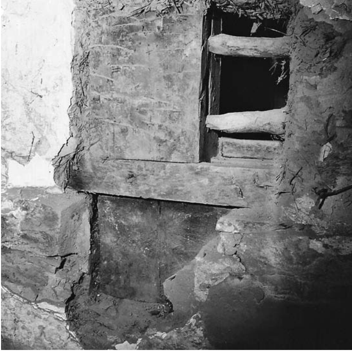
Fig. 5 – Detail of exploratory opening showing the end of a first floor beam; 3 by 6 inch sill let into the end of the beam; lower portion of a wall post showing hacking of its outside surface to hold plaster. Horizontal sticks set on about 6 inch centers to hold infill of clay bound with straw. October 1969.
