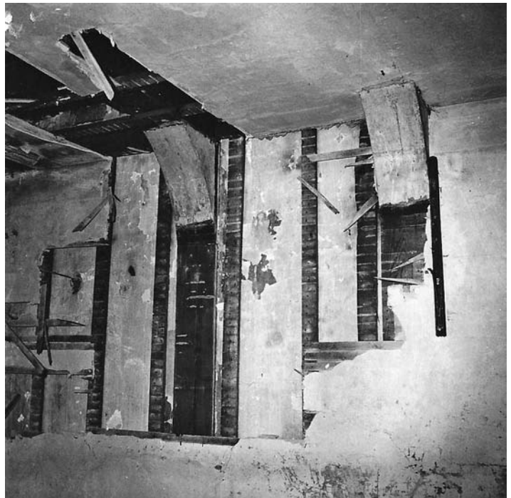
Fig. 12 – Interior of the south wall, first floor, of the North House at an early stage in the removal of the 1878 lath-and-plaster work. At this stage, most of the ceiling plaster was still in place. Note how the 'korbeels' were left protruding into the room space, and their exposed portions were whitewashed along with the plaster. September, 1969.
