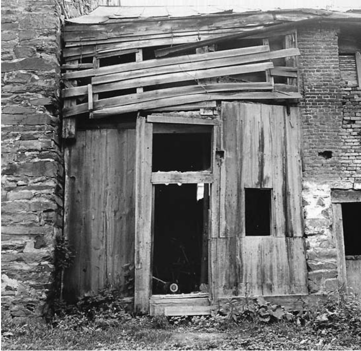
Fig. 1 – East elevation of the 'connector' between the Coeymans mansion and the North House. September 1969. All photos by J.R. Stevens.
