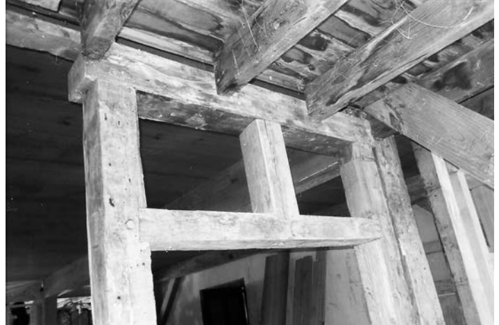
Fig. 4 – View of extant door frame in Ten Broeck House. Photo by author.
