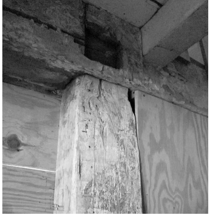
Fig. 6 – View of post in center partition (now west wall of center passage) with empty mortise for trimmer beam in beam above and ghost of jambless hood molding. Photo by author, 2014.
