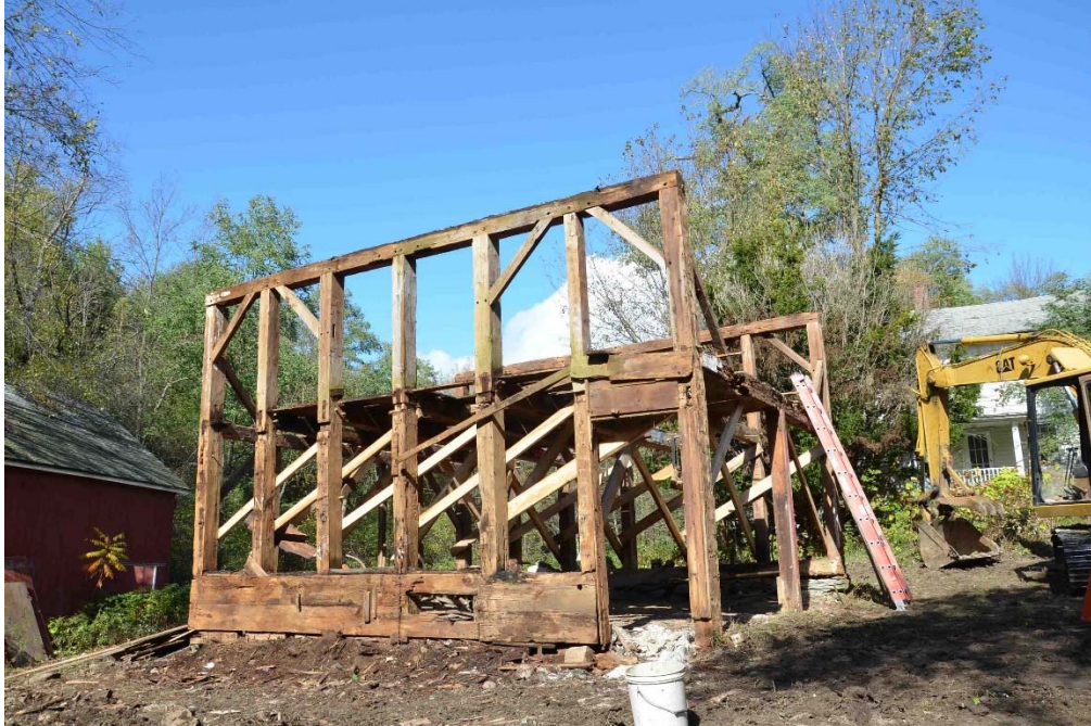
Figure 10. The Gibbs barn in the process of being disassembled (photo by Connie Kheel, 2012).
